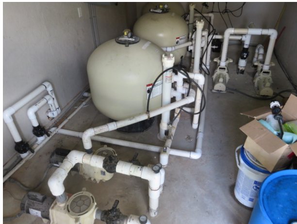
Pool mechanical equipment
