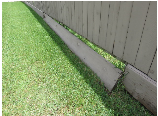
Base board deterioration and displacement
