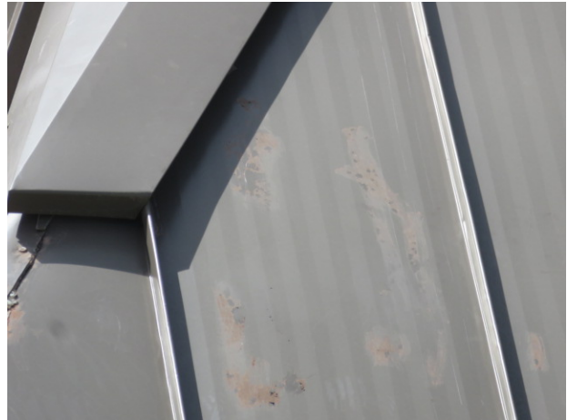
Roof rust at standing seam panel
