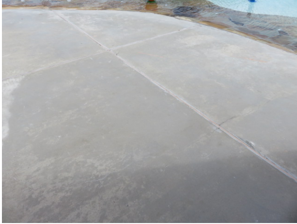
Pool deck in good condition with isolated and minor deterioration
