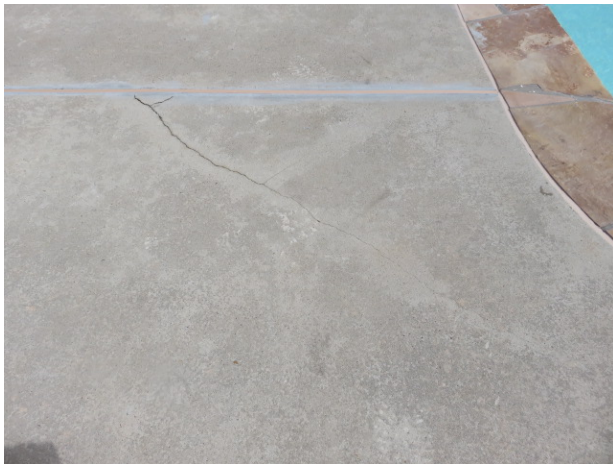
Isolated pool deck crack
