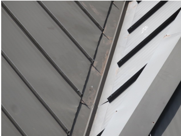
Roof rust at valley
