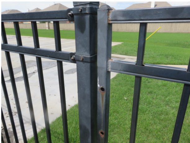
Rust and finish deterioration at pool fence
