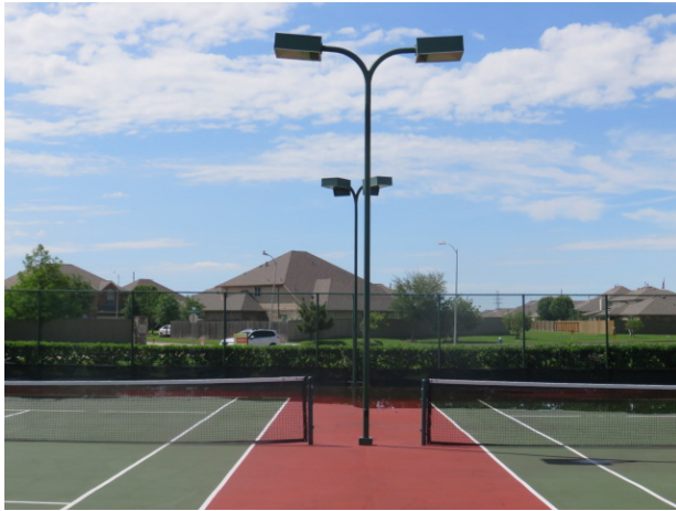
Light poles and fixtures
