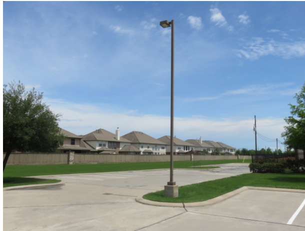
Metal light pole and fixture at amenity center
