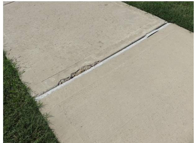
Isolated concrete sidewalk deterioration along joint
