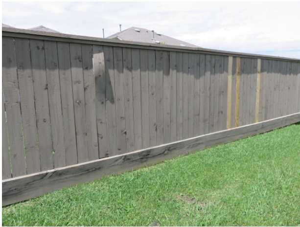
Fence board warp and partial replacements
